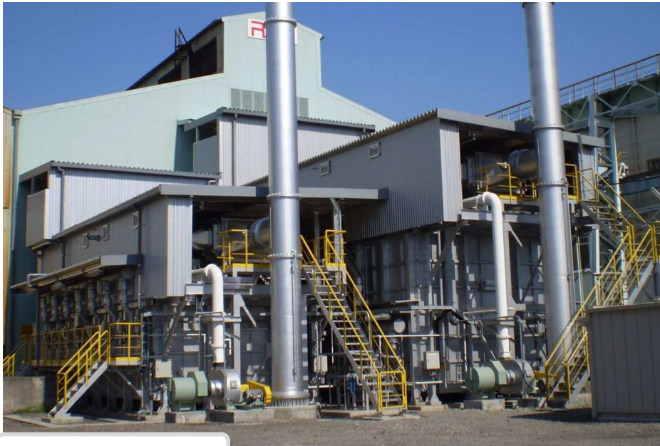
Heat Treatment Furnace
